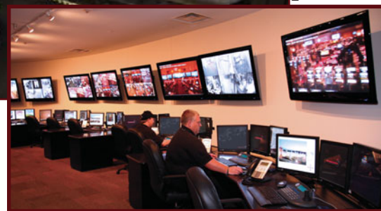
Hollywood Casino's new control room, one of the most advanced in the country, supports up to nine operators and two supervisors at any time. The command center features a touch-screen control interface and IP Video Wall.
