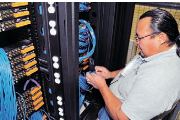
Daryll Mouse of Technical Security Integration (TSI) wires up the paddleboards for Synectics' internal PCI-e 16-channel encoders.
